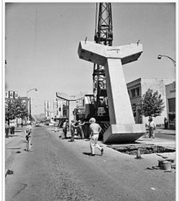
Building the Seattle Center Monorail , 1961. Looking north up Fifth Avenue from Virginia Street.
